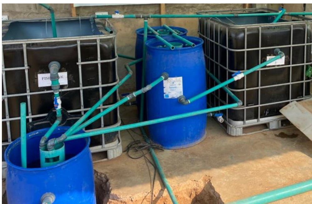
Figure 3: Filter connected to the overall system
