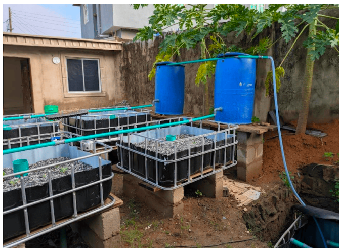
Figure 2: Photo of implemented system at ADC, Lagos, Nigeria
